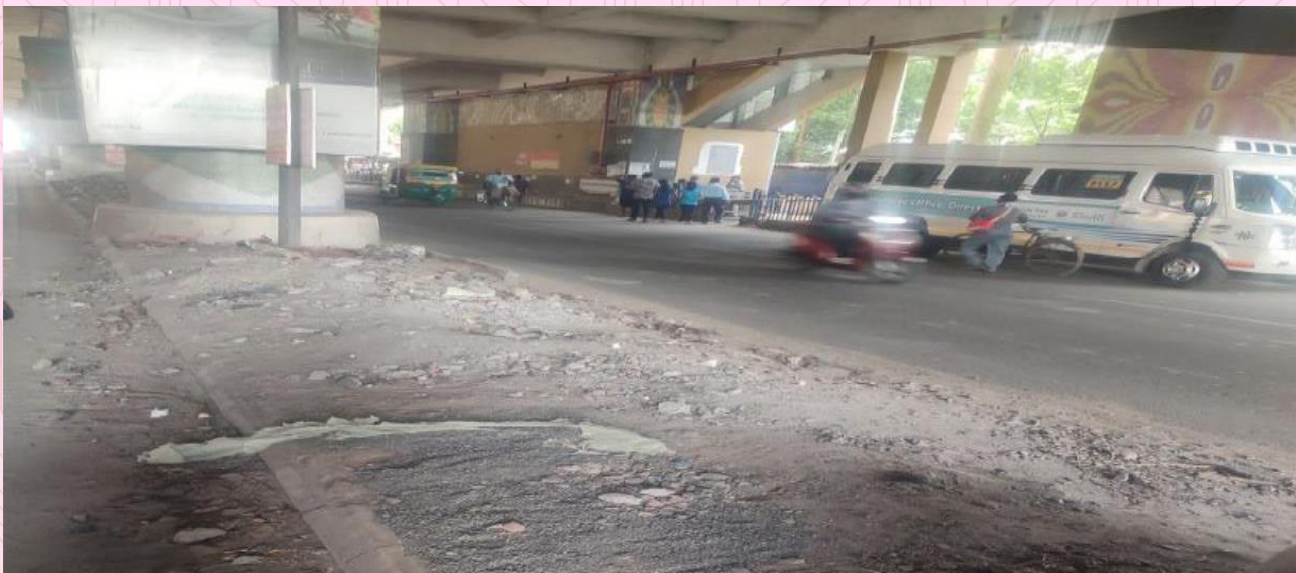
Broken Bamboo Fencing (Before)
